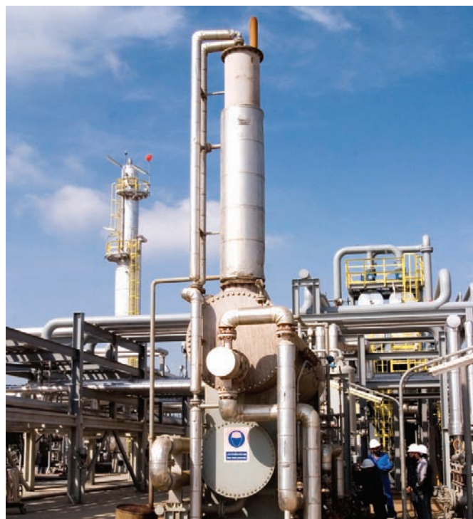
A team of engineers inspect the Dana Gas processing plant in Egypt.
